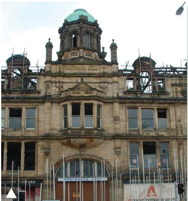
Eastbrook Hall, formerly the Methodist Cathedral of the North, built in 1904, suffered a major fire in 1996 leaving it derelict, burnt out and roofless
