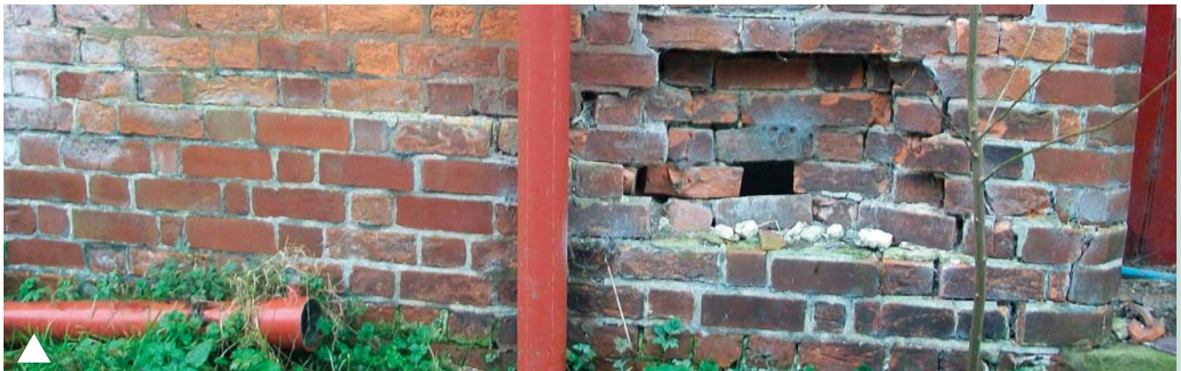
Brickwork damage and poor repair
