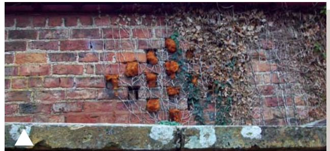
Inappropriate blocking up of historic feature of farm building
